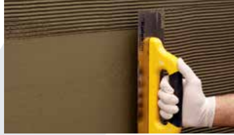
Application and raking of the 1st coat of Mantoplast thermal insulation board plaster mortar.
